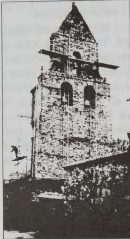
Work in progress on the tower at Rabanal del Camino in April 1999. Photo: Howard Nelson.
