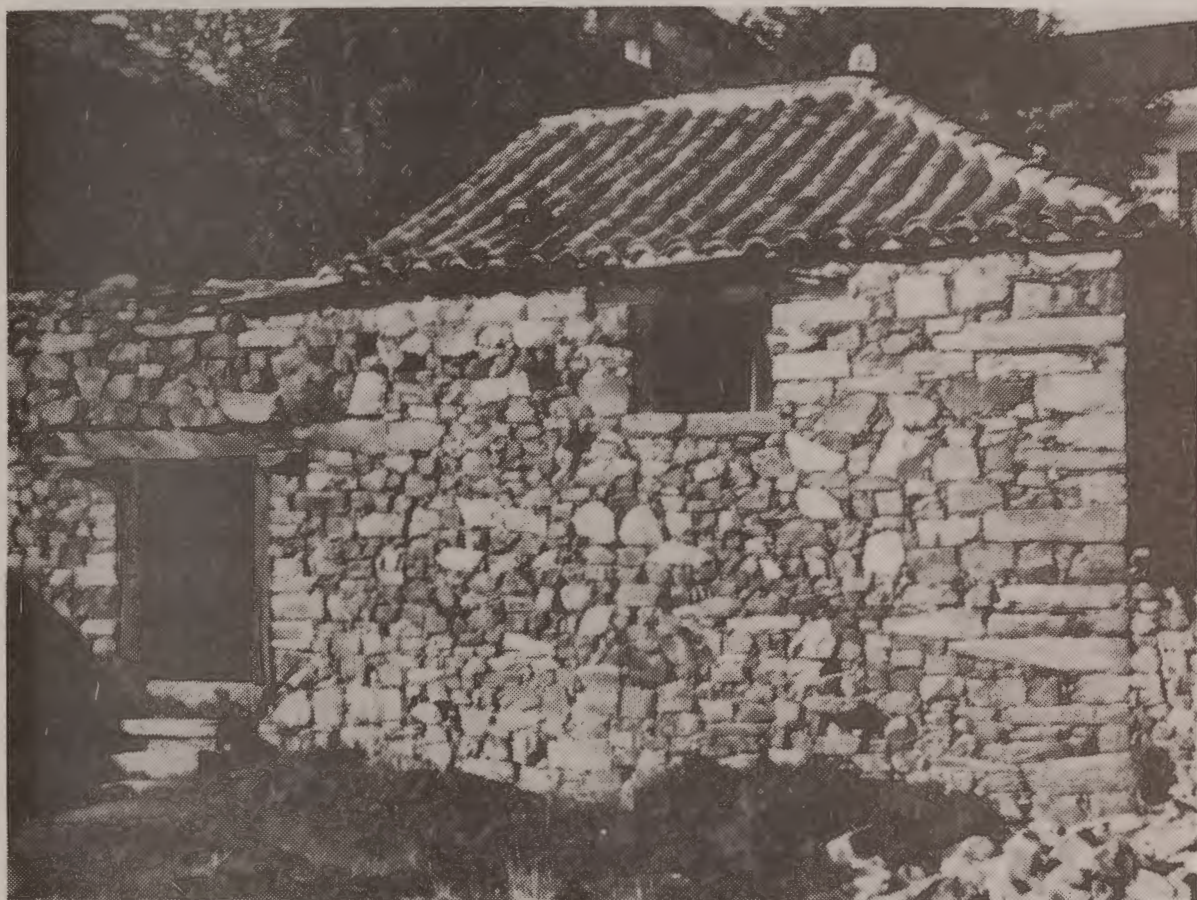
Rear of Barn with 'New' Roof and Rebuilt Walls. Photo: Charles Francis
